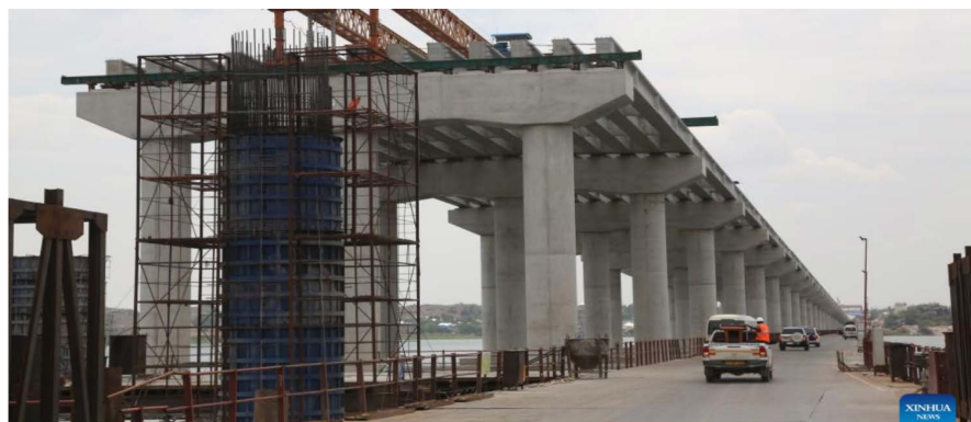
Figure 1. Construction of John Pombe Magufuli Bridge over Lake Victoria in Mwanza region undertaken by China Civil Engineering Construction Corporation (CCECC) and China Railways 15 th Bureau Group which is also under Built and Road Initiative (Photo by Herman Emmanuel/Xinhua Sep 9, 2023).
