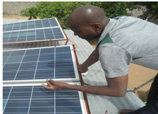
Fig. 1. Trees debris and bird's droppings are accumulated on the surface of PV modules (Visual Inspection)
